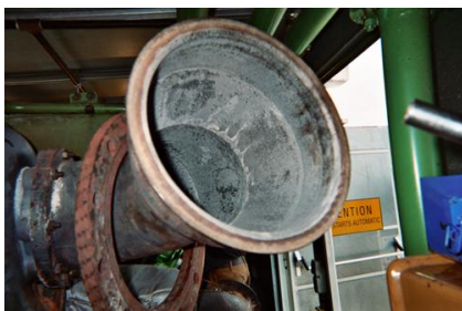
Siloxane deposits in engine exhaust line
